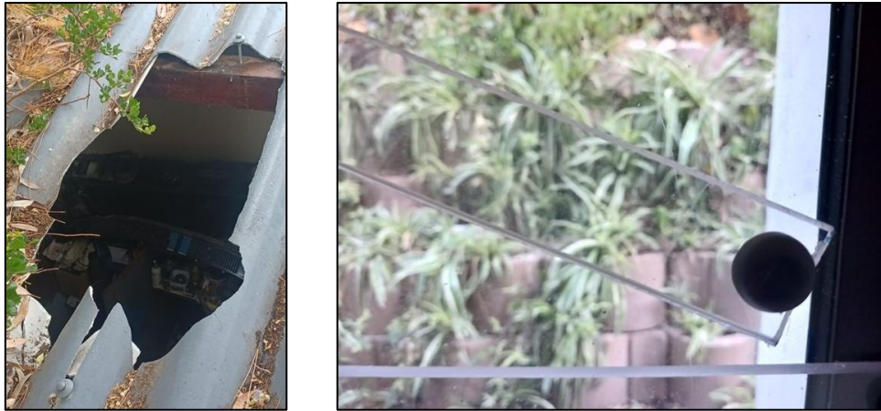
Figure 2. An outbuilding roof in Da Gama Park which was inadvertently damaged by baboons while playing/fighting (left) and burglar bars which were broken by baboons in Simon's Town (right).
